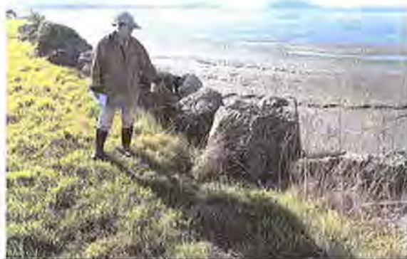
Photo 4 – View southwest showing erosion occurring at top of dike approximately 2.5 feet landward of MHHT/OHWM.
