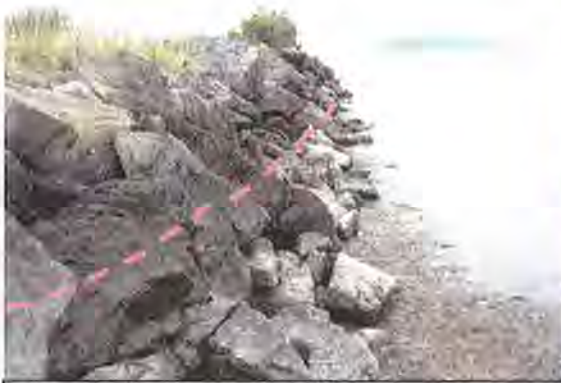
Photo 3 – View of rock face of dike showing detritus at toe, lichen and approximate 8.4' elevation of MHHT at dashed line.
