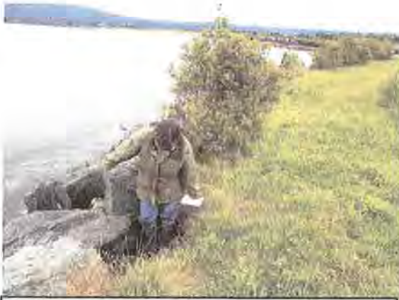
Photo 3 – View north showing eroded area proposed for repair along waterward top of bay front dike.
